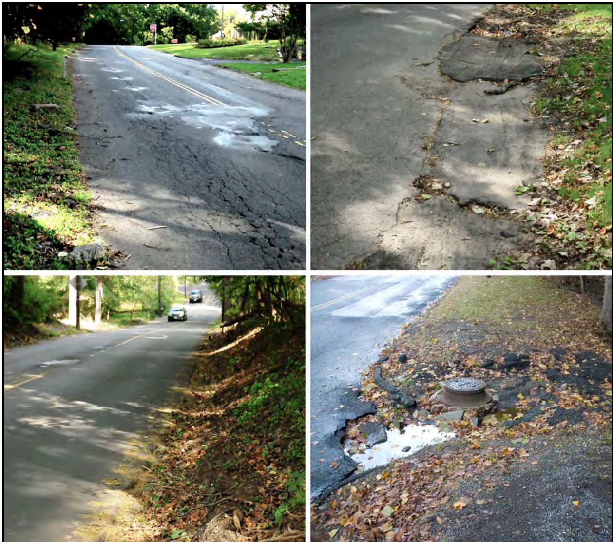
Figure 1-2. Deteriorated Infrastructure along Oregon Avenue
